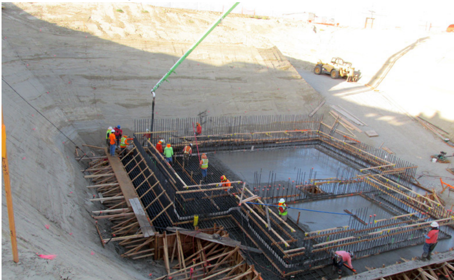
Coachella Valley Water District Headworks, Plants 4 and 7 | Indio and Thermal, California
